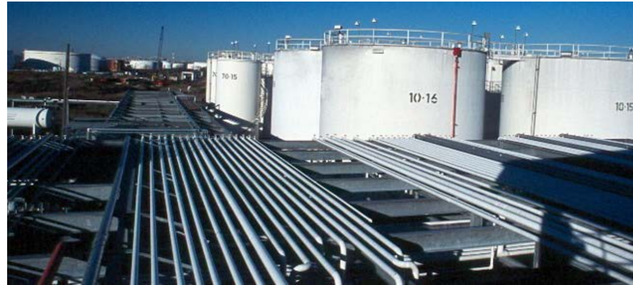
Solvent and Resin Storage
